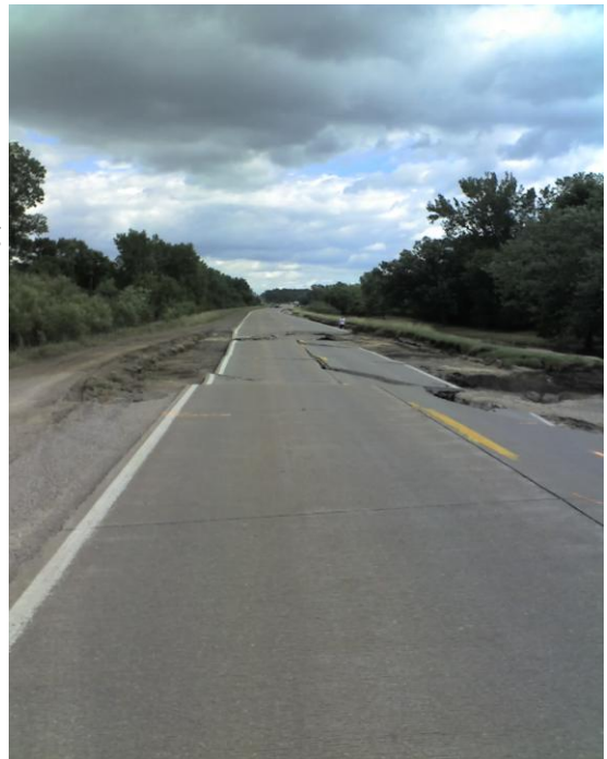
Flood damaged road in eastern
